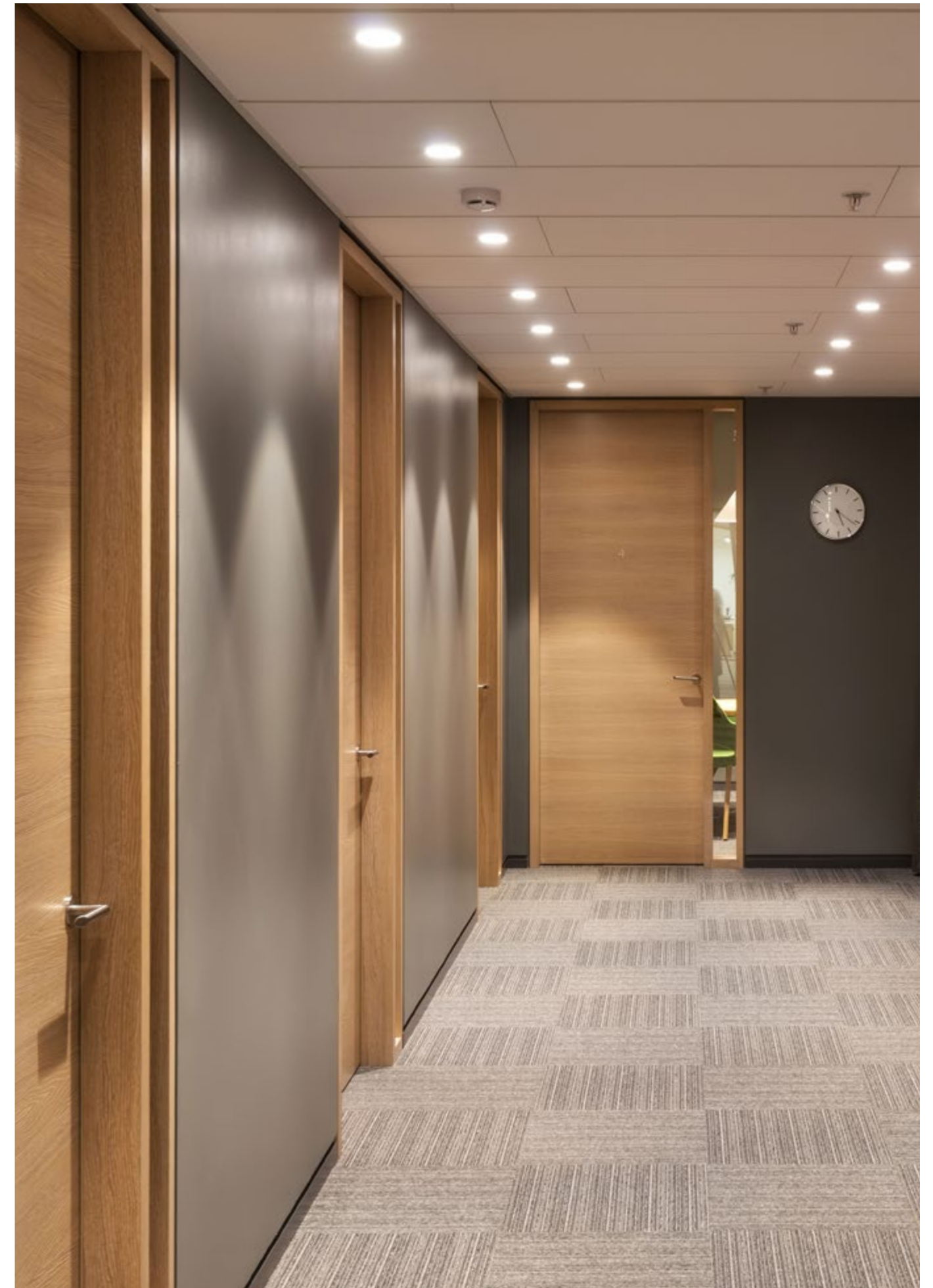
Application of RQ 160 LED in corridor.
